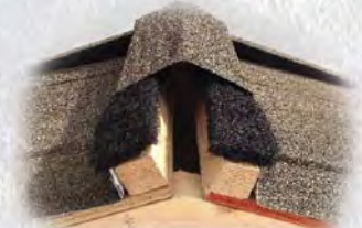
Installed without Center Beam
